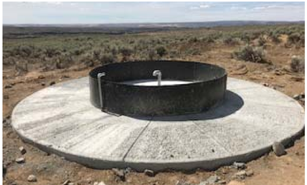
Livestock water facility with concrete pad.
