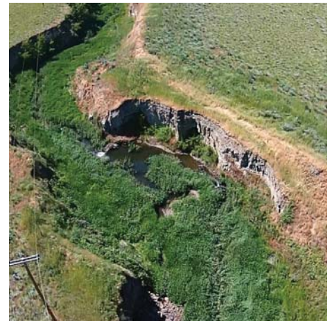
First beaver dam analog installed in 2015. Since then, 100 have been installed on Lower Pataha Creek. Photo by Duane Bartels
