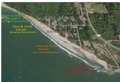
North Cove Dynamic Revetment Phase 2 West Project to start construction Fall 2018 and be completed by spring 2019.
