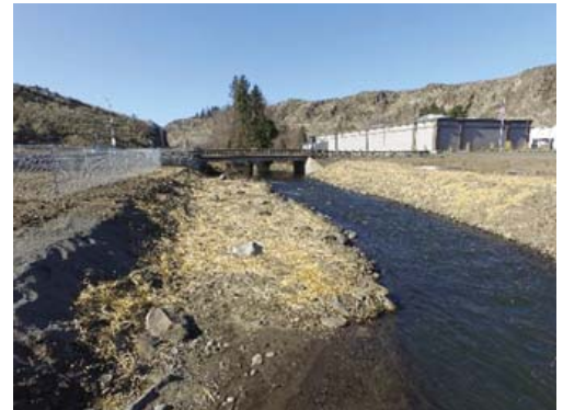
Finished project showing replaced siphon and reconstructed streambed. Photo by Justin Bader
