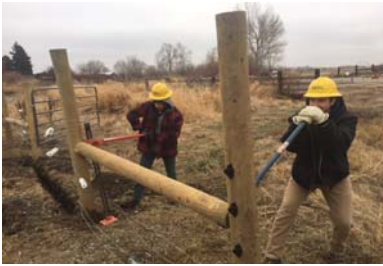
NYCD's Washington Conservation Corps crew building livestock management fencing at Ahtamun Creek - Field's Project. Photo by Brian Schmidt
