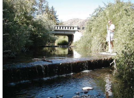
Exposed siphon creating fish passage barrier during low flow. Photo by Mike Tobin
