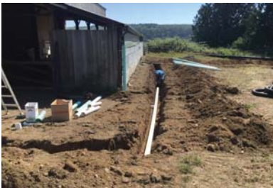
Downspout drains being installed to divert stormwater from livestock pasture and prevent manure from entering Discovery Bay.
