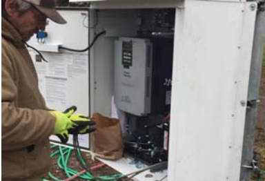
Installation of a new variable frequency drive controller. This new technology conserves water and energy.
