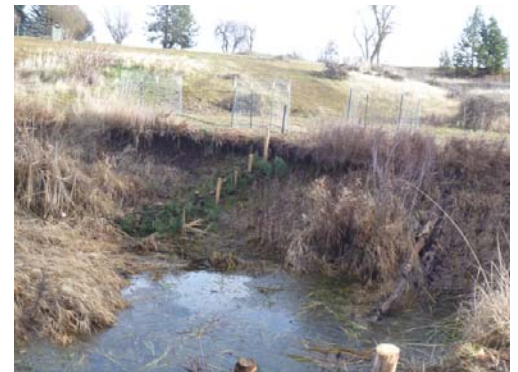
Post assisted wood structure with willow plantings along the streambank and enclosed native trees and shrubs planted above.
