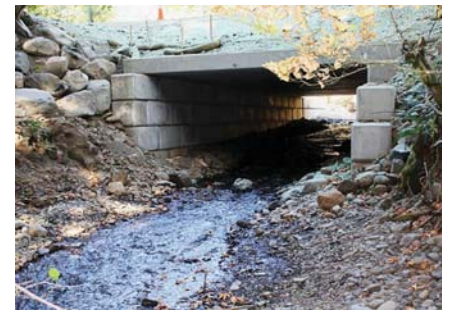
The newly constructed modular box culvert with a constructed streambed to simulate a natural stream for fish.
