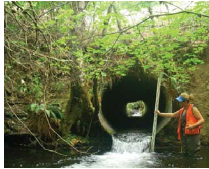
Former fish barrier culvert under Lakeview Road, considered a 100 percent barrier due to its slope and outfall drop.
