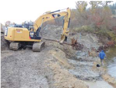
Streambank stabilization on the Colville River will reduce sediment and protect productive agricultural ground.
