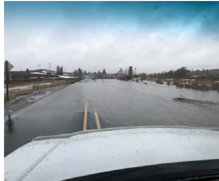
Flooding on SR27, with Oakesdale beyond and sewage treatment lagoons immediately to the left of picture.
