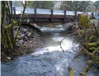
Fronia Creek – before (top) and after (bottom) fish barrier was replaced with bridge.
