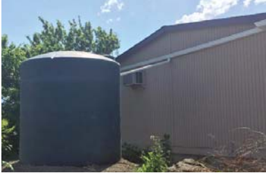
Assisted Sequim High School with installation of a roof water collection demonstration project.
