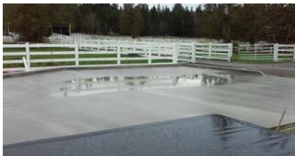
After: Concrete waste holding structure has curbs to prevent run-off and will allow the stable to house bins for manure holding until haul-off.
